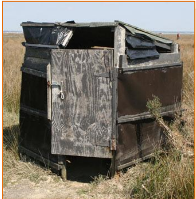
Figure 56 : Cabinet WC isolé
